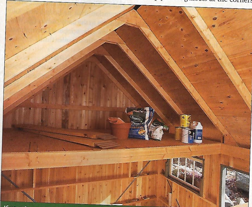
If you choose, you can customize the shed by creating a small storage loft at one or both ends. Here, the 2 x 6 chords of central trusses are cut away after assembly and their cut ends are framed across. Then, a plywood deck is installed.
