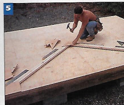
5 Assemble all of the roof trusses on the shed floor. Nail plywood gussets across the joints on both sides of the trusses.
