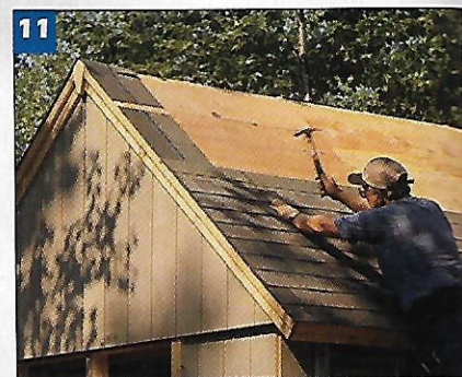
11 Cover the plywood roof sheathing with asphalt shingles. Eight bundles are needed to complete this roof.
