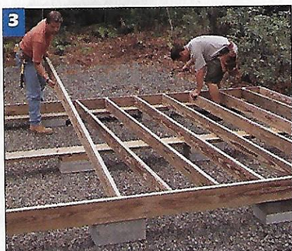
3 Install a 2 x 6 floor joist every 16 in. Fasten them by nailing through the band joists with 16d galvanized nails.
