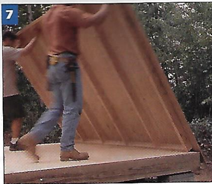
7 Carefully raise the end wall into position. Note how the plywood siding hangs down to cover the floor framing.
