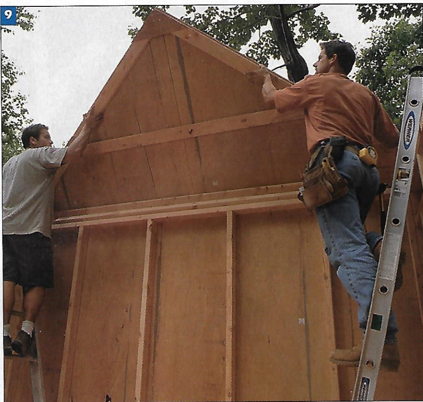
9 Start the roof by installing the end trusses. Note that the plywood siding is nailed on before the truss is raised. A central 2 x 4 chord stiffens the sheathing.
