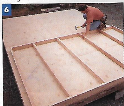
6 Build the exterior walls on the floor. Assemble the 2 x 4s with 16d nails and then add the plywood sheathing.
