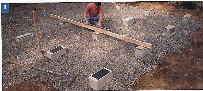
1 Use a 4-ft. level and a long, straight 2 x 4 to ensure that the concrete foundation blocks are level. Add shims to build up any low blocks.
