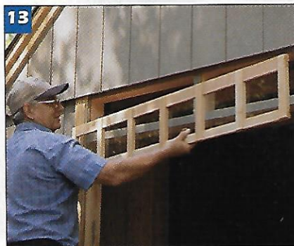
13 Make the 5-ft.-long transom window from a wooden frame and a single piece of glass. Install it over the end doors.
