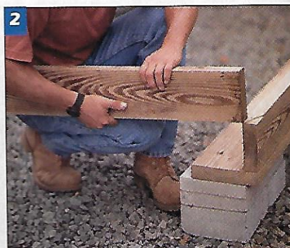
2 Set the 2 x 6 floor joists on top of the 2 x 8 mudsills. These floor-frame parts are cut from pressure-treated lumber.
