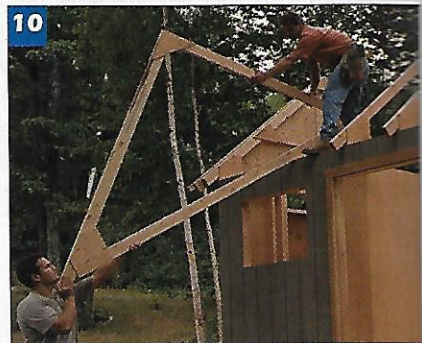
10 Carefully slide the roof trusses onto the walls. Space them 24 in. on center and secure them with 3-in. screws.
